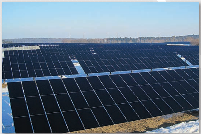
5600 kW in Jatzke, Germany, December 2010
